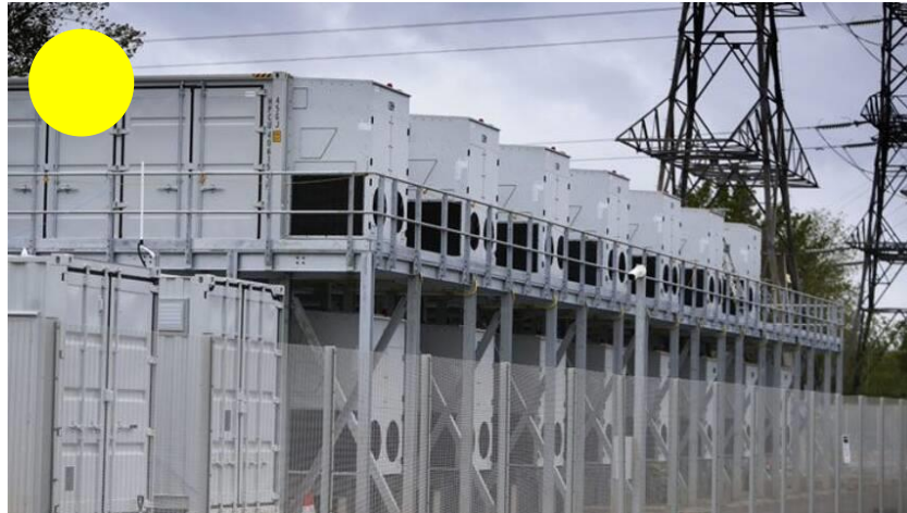
Energy Storage - Batteries (Industrial Scale Batteries)
