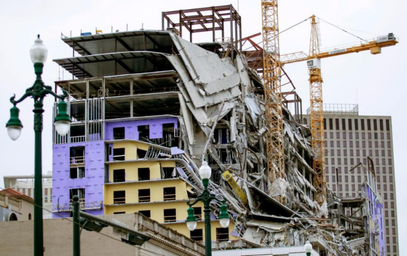
New Orleans Hotel Construction Collapse, 2019
